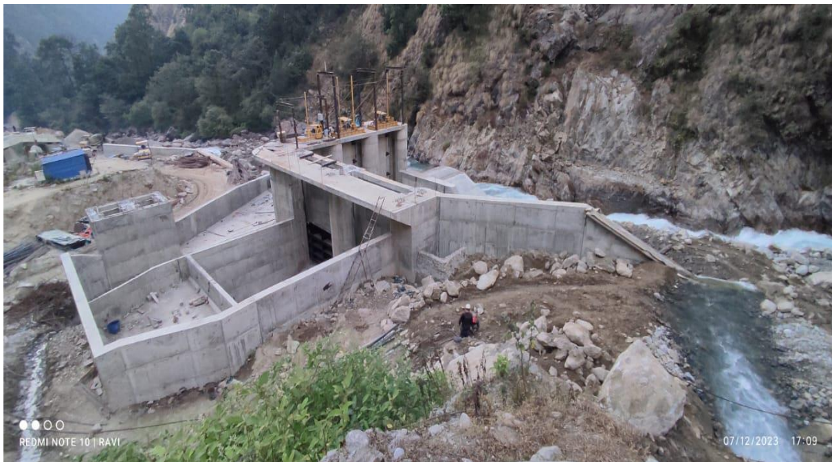
Figure: Headworks area
