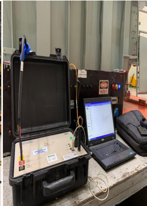
Figure SFRA test of power transformer
