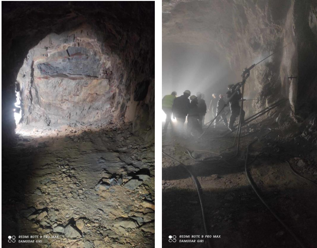
Figure: Surge Tunnel
