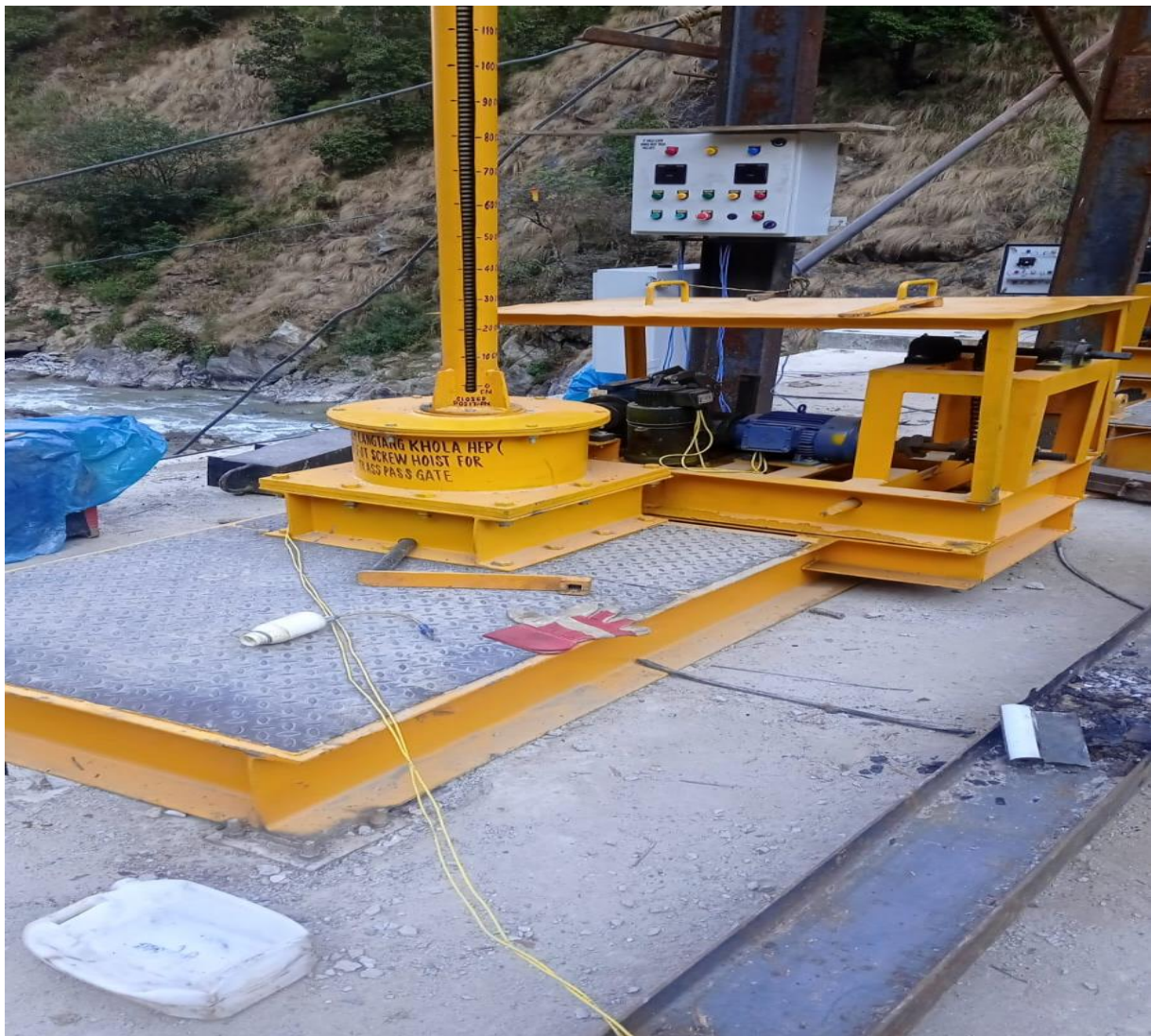
Figure: Trash Pass screw hoist with control Panel arrangement
